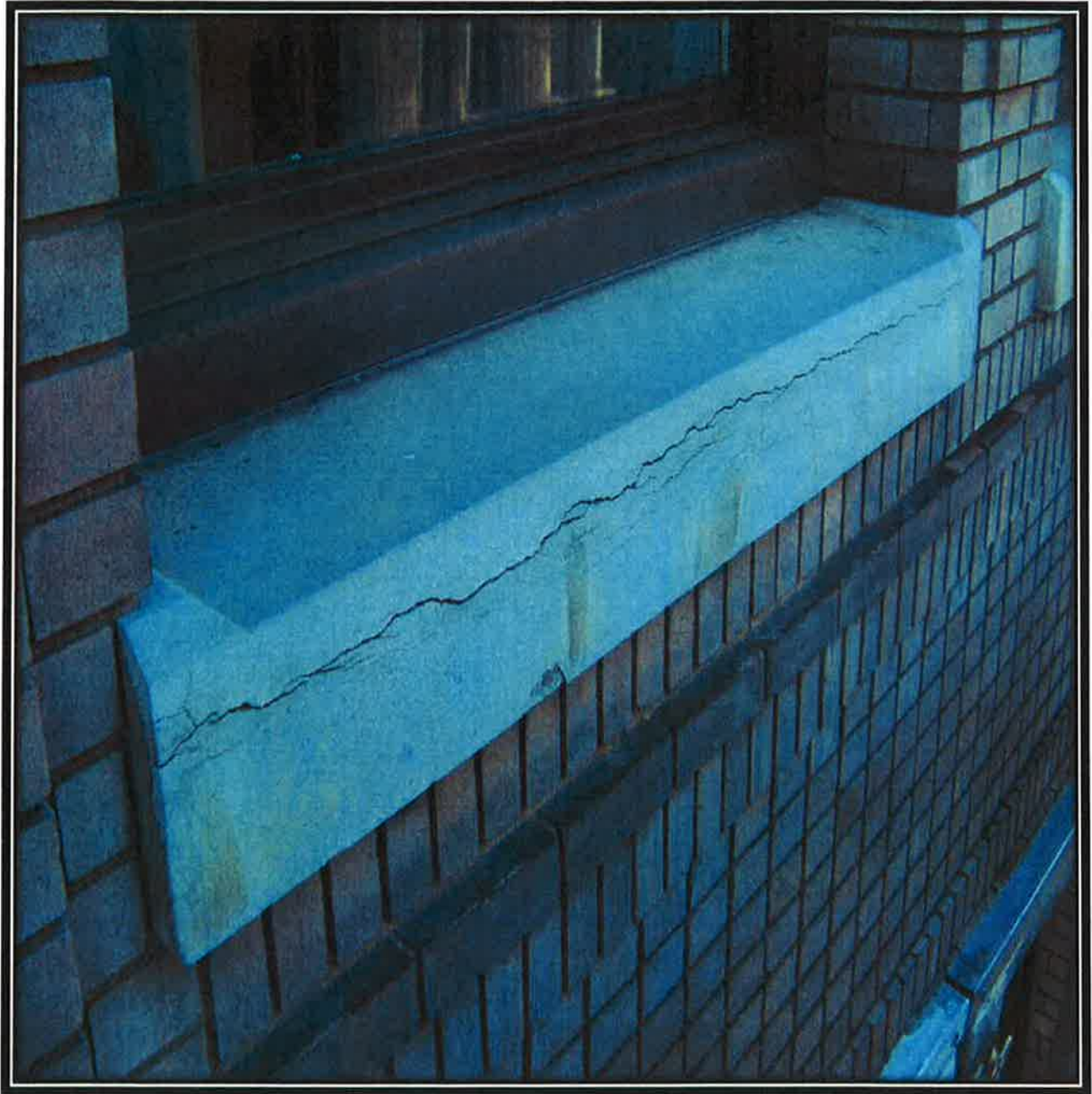
Cracked window sills to replace with limestone
